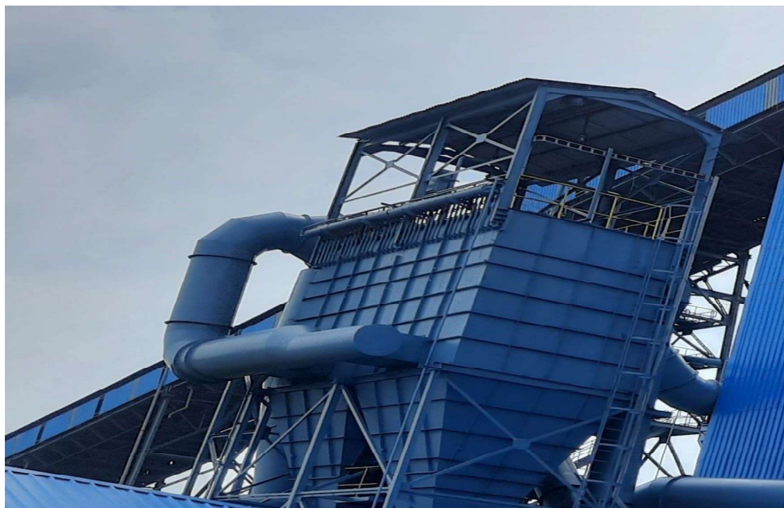
DUST EXTRACTION SYSTEM AT TRANSFER POINTS
